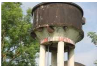
Small water towers, Rampur campus
